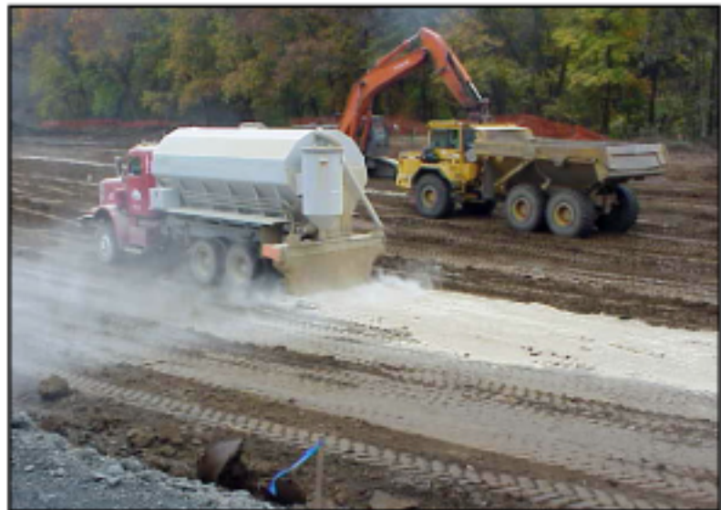
Ash Grove Durabase® CKD is placed onto the soil for stabilization at the Monticello Dam Project in Lenexa, Kansas.
