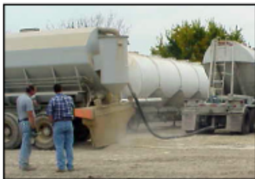
Ash Grove Durabase® CKD is transferred from the delivery truck to the spreading operation.
